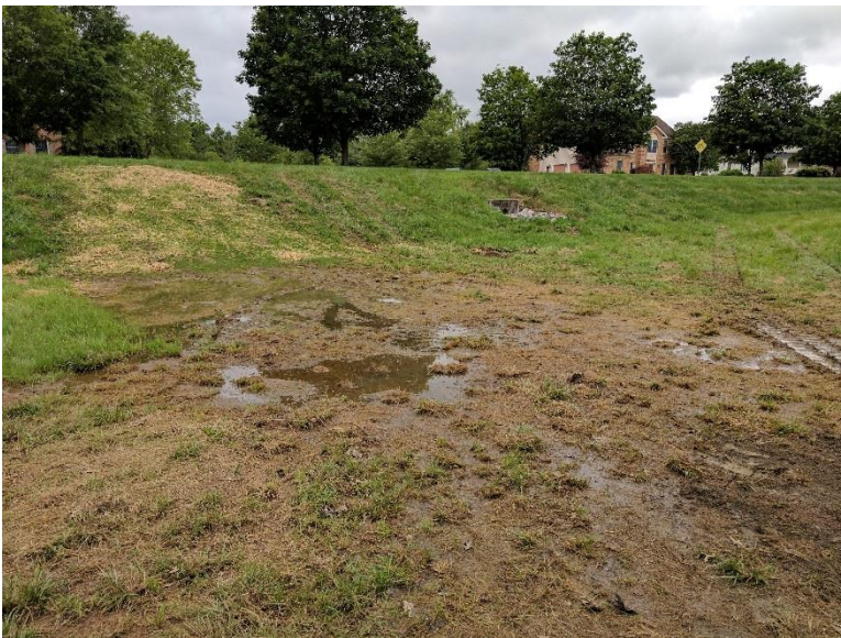
Photo 23 The embankment area that had already been disturbed on 5/22 was further disturbed 6/7/17. There was a light rain which would have increased soil compaction
